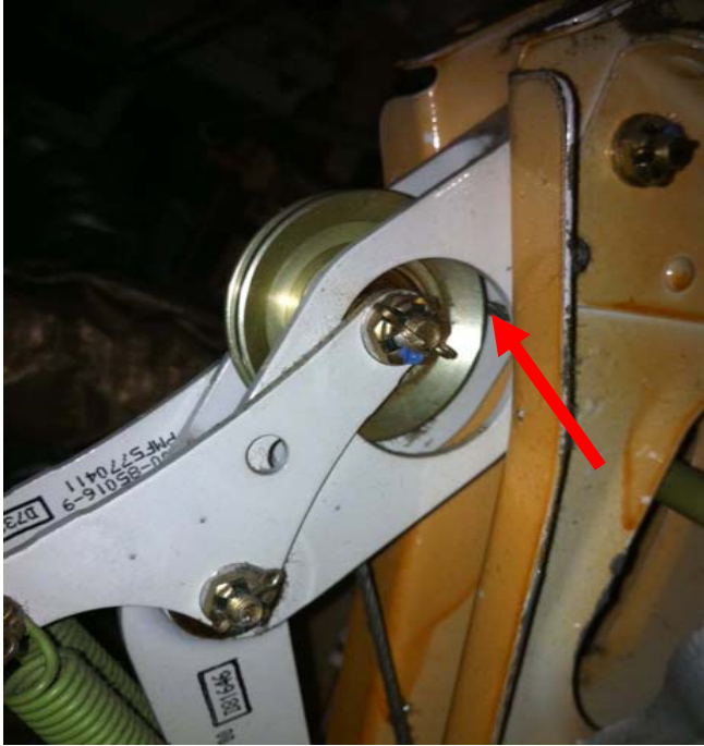
Manual gear release under-floor pulley lever system with a jumped and jammed cable.
